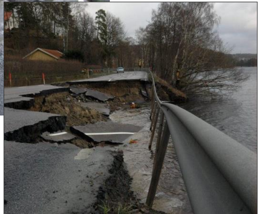
Storm damage, northern Sweden, late September 2011
