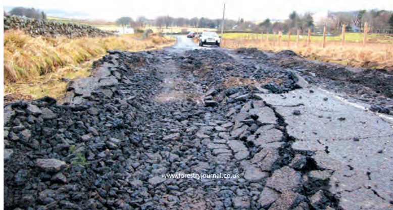
Damage caused by frost heave.
